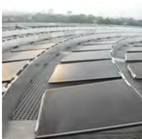
Figure 151: Installation with thin-film modules
