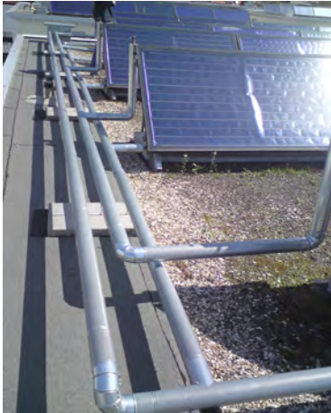
Figure 251: Mineral wool with a metal sheet casing
