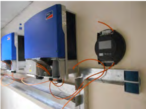
Figure 206: Data wiring of inverters and control device (SolarLog)
