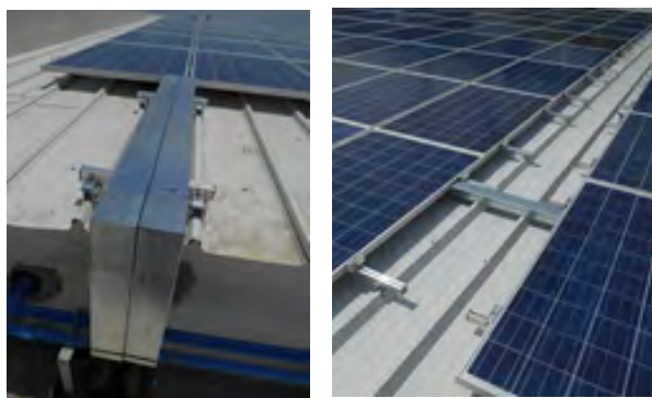
Figure 203: Cable duct for DC wiring on the roof and AC wiring at the inverter
