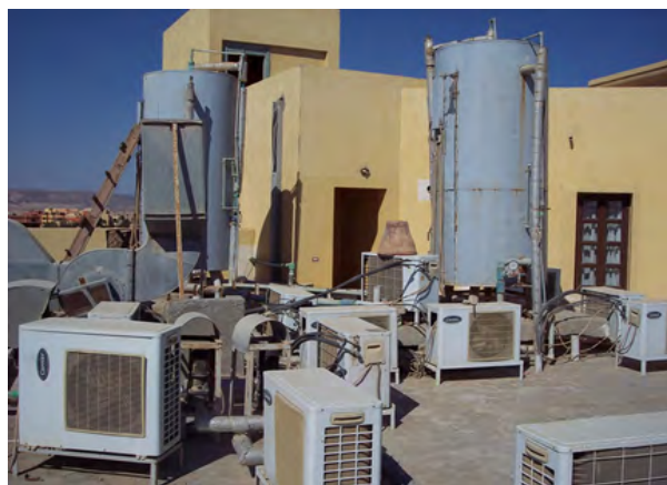
Figure 270: Defect storage tanks and electric heaters.
