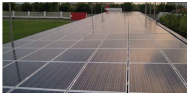
Figure 18: Installed PV modules
