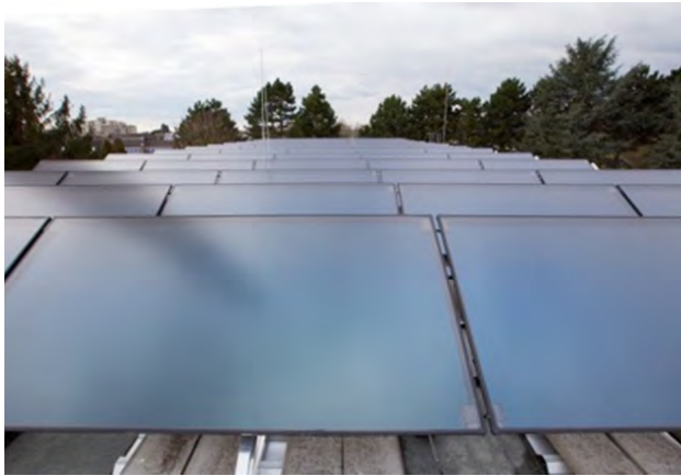
Figure 36: Solar thermal collector
