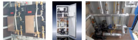
Figure 239: Pre-assembled module to transfer the heat to the storage
