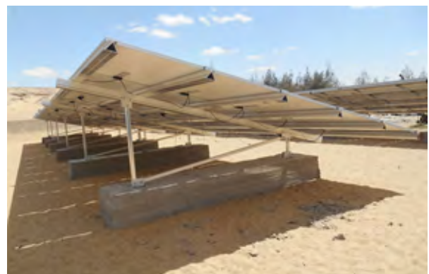
Figure 164: Solar on-ground installation with concrete foundations in Bahariya, Egypt
