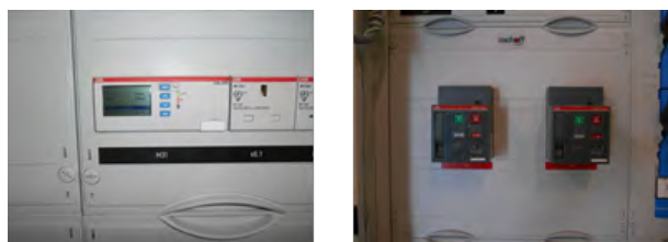
Figure 184: Grid and system protection with monitoring relay and motor switches
