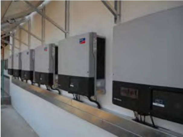
Figure 17: Inverters in a solar power system
