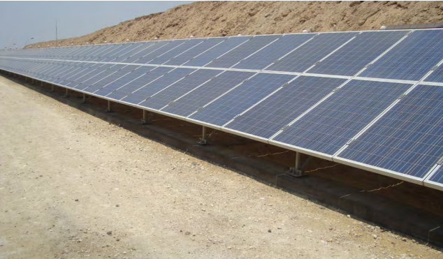
Figure 66: Open area solar power system
