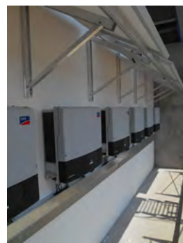
Figure 198: Inverter installation under a solar panel roof for shading
