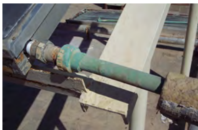
Figure 267: Wrong piping material for hot water or solar installation
