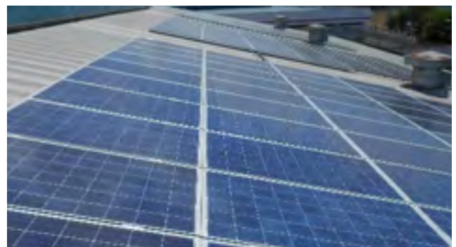
Figure 149: Installations of polycrystalline modules
