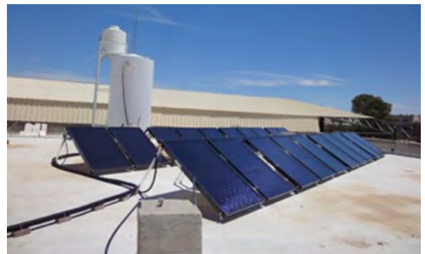
Figure 12: Solar power and solar thermal systems
