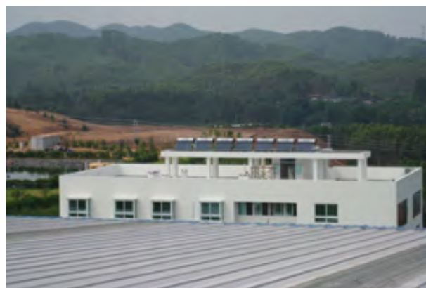
Figure 56: Multi-Solar Water Heater system for smaller hotels
