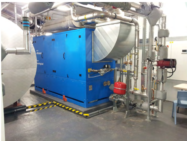
Figure 96: Combined Heat and Power unit
