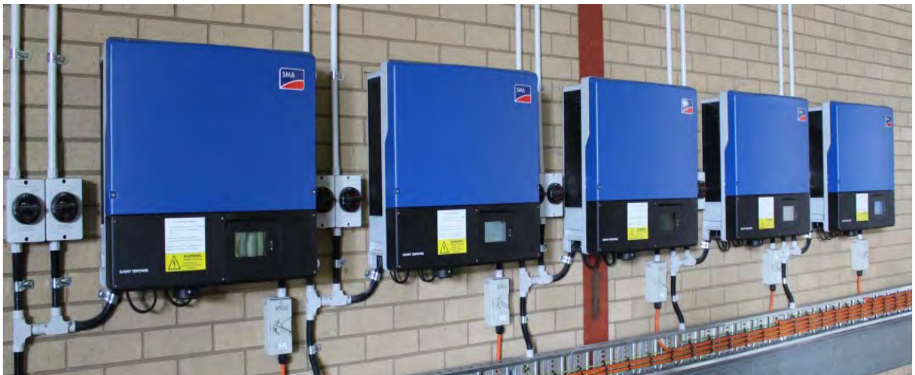
Figure 25: Solar inverter installations
