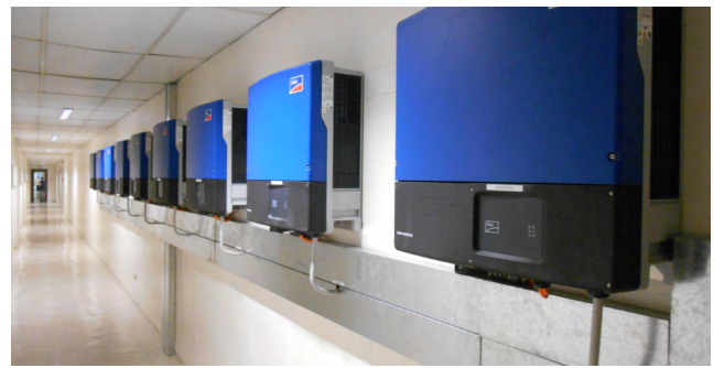
Figure 132: Typical string inverters with strings directly connected to the inverter
