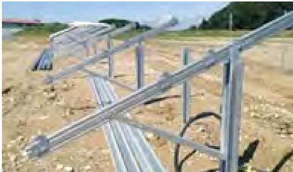
Figure 165: Solar on-ground installation with pile foundation
